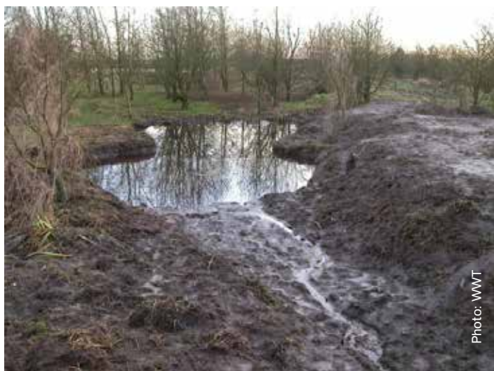
Figure 11. Newly created sediment pond with clay lining as part of a constructed farm wetland.
